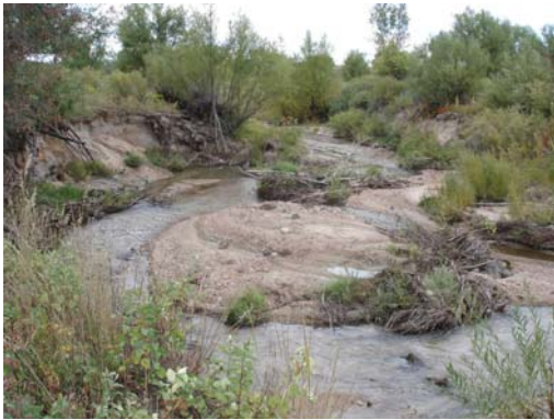
Bank erosion along E. Plum Creek
